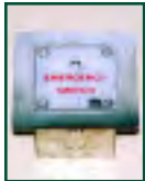
Fireman's override switch
