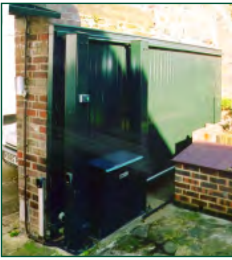
Gate in open position with view of control box
