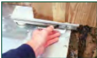
Manual release for Earth Operator This essential safety feature is very easily accessible should it be necessary to release the gates.
