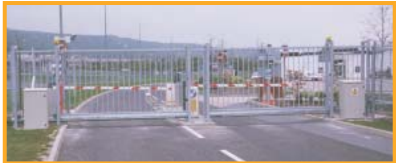
Pair of Sentry cantilever automatic sliding gates plus auto-barriers
