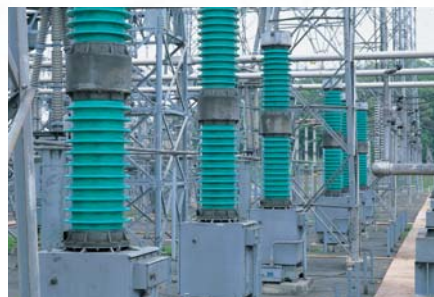
Protecting insulators from salt-air
